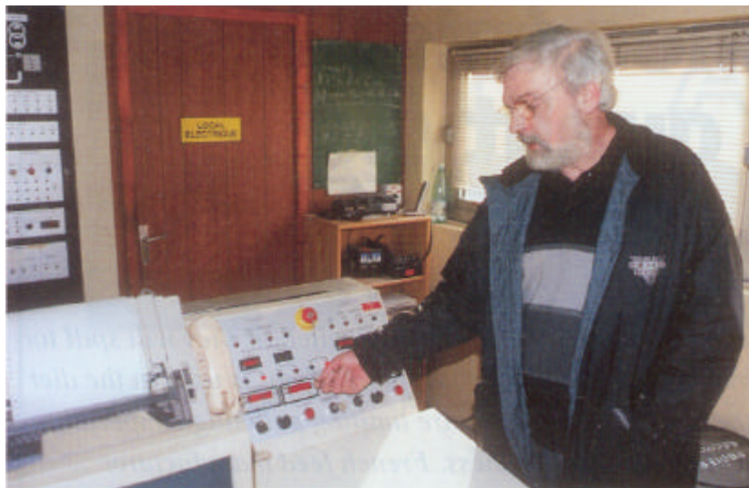
In the control room a separate control panel is installed to manage the process. Jean-Pierre Peire points out that control of the system is very important.
